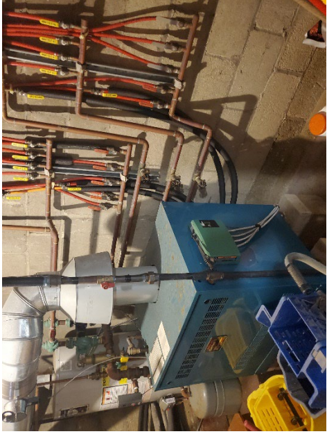
Photo 14: View of the gas-fired boiler, its related piping manifolds, and adjacent domestic water heater that serves the Church portion of the Building and is located in the Basement. Such equipment should be relocated to the 1 st Floor
