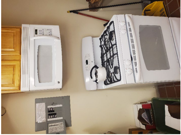
Photo 13: View of an electrical subpanel within the Kitchen area of the Basement of the Church that should be eliminated. Note also the gas stove, which should be replaced with an electric induction type unit.
