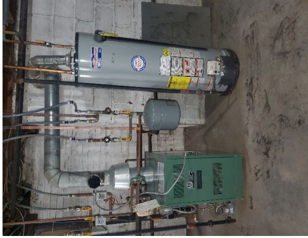
Photo 15: View of the gas-fired boiler and domestic water heater that serve the Rectory portion of the Building and are located in its Basement. This equipment should be eliminated and the loads served by new equipment located above the design flood elevation.
