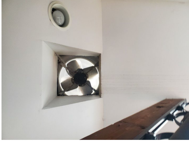
Photo 24: View of an exhaust fan in the Church Overcroft that should be removed and the opening sealed.
