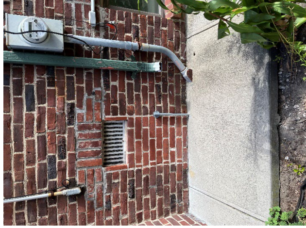
Photo 40: View of the electric meter for the Building. The upgraded replacement should be raised to about 60" above the walkway. Also note the outdoor air intake to the Church Boiler Room referenced in photo 26.
