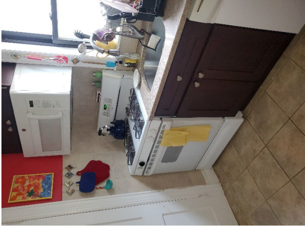
Photo 16: View of the gas stove within the Rectory Kitchen. This unit should be replaced with an electric induction type stove.
