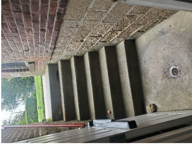
Photo 5: View of the exterior stairs serving the Church Basement. Note the floor drain, which appears to be connected to a dry well.
