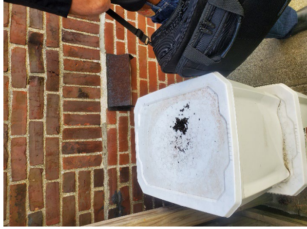
Photo 39: View of an open vent, typical of several. Such vents should be relocated or sealed if not needed.
