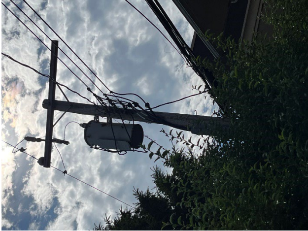
Photo 9: View of the electric service transformer serving the Building and others. This is located near the southeast corner of the Building. The transformer will need to be replaced and upgraded 400A capacity to serve new loads.
