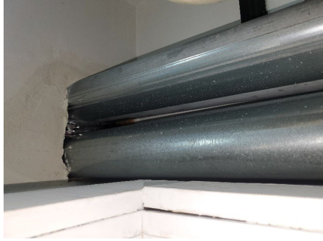
Photo 36: View of duct risers extending down to 1 st Floor through a 2 nd Floor closet. Note that the opening is unsealed and the ducts uninsulated.
