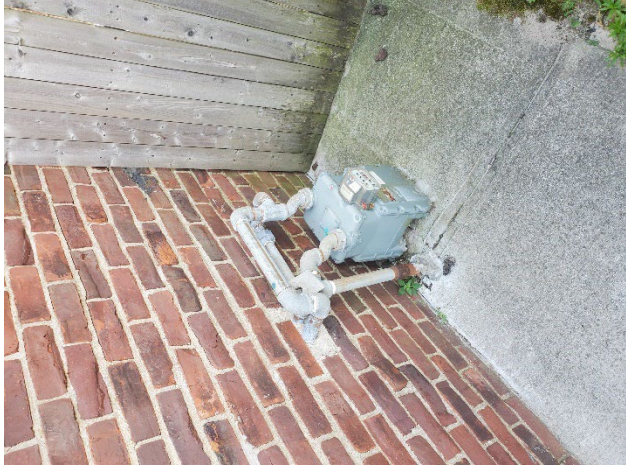
Photo 10: View of the gas meter, which is located at the southwest corner of the Building. If retained, the gas meter should be raised to be 48" above the sidewalk.
