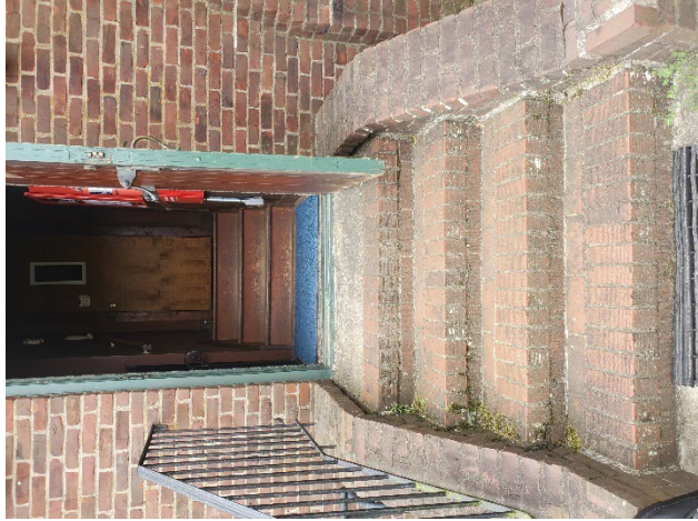
Photo 3: View of the exterior and interior stairs leading to the Church. At the intermediate interior landing, stairs to the left lead down to the Basement.
