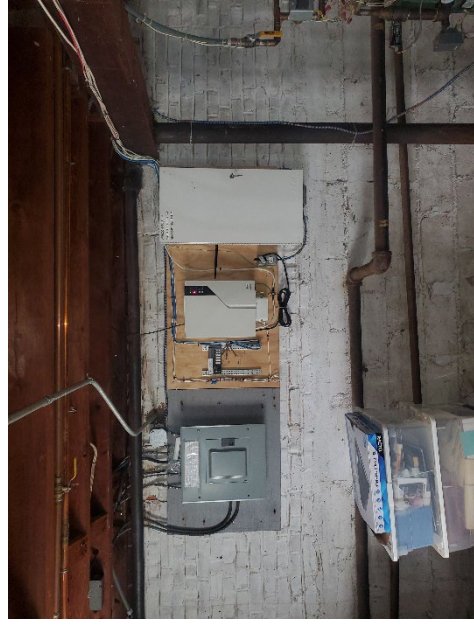
Photo 12: View of the electric subpanel that serves the Rectory portion of the Building and is located in its Basement. Also note the adjacent telecommunications panel. The subpanel should be relocated to the 1 st Floor of the Rectory. The telecom equipment should be relocated to the Church due to space considerations.
