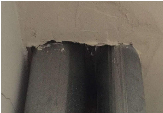
Air conditioning duct in 2 nd floor of rectory going to attic
