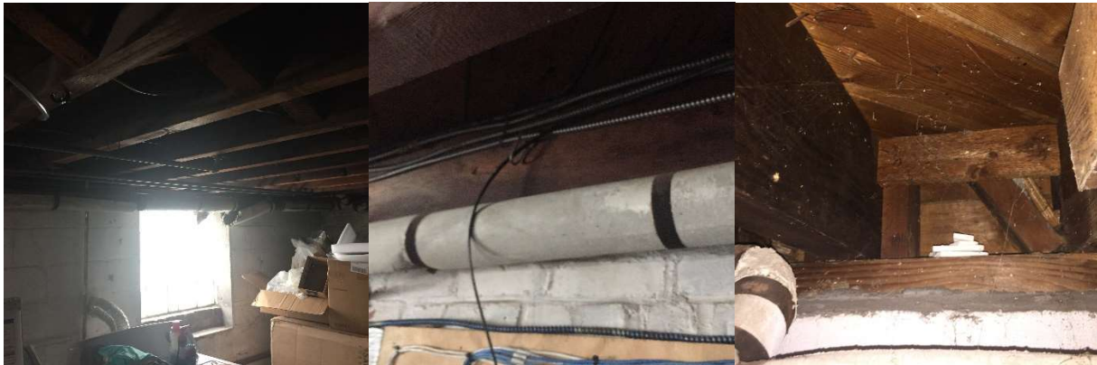
1) Rectory basement showing joists where they meet foundation wall;2) last joist on the end, running along foundation; 3) rim joint pocket between joists at wall (concrete basement wall at bottom)
