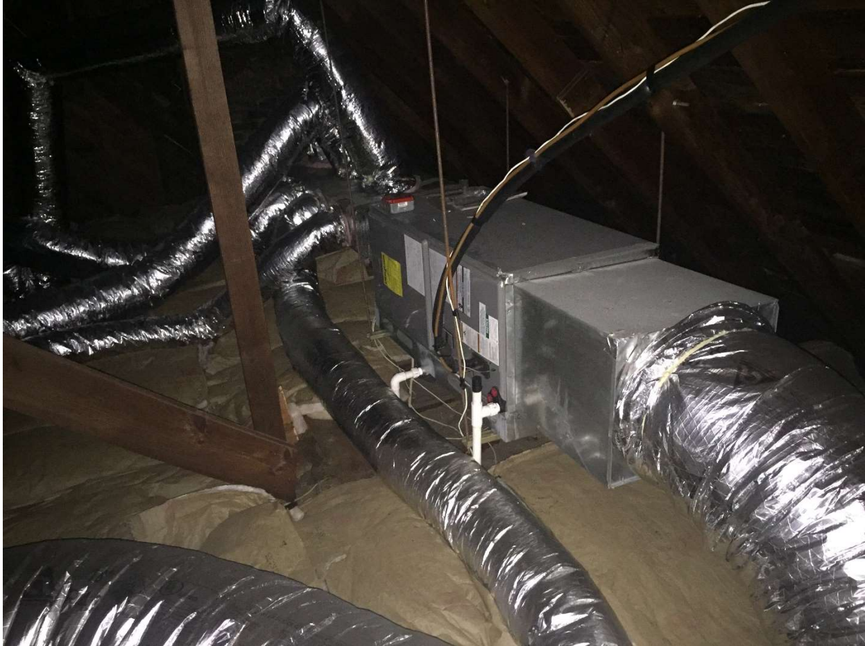
Rectory attic air handler with insulated ductwork serving the second and first floor of the rectory
